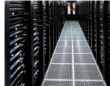
Telecom base station
